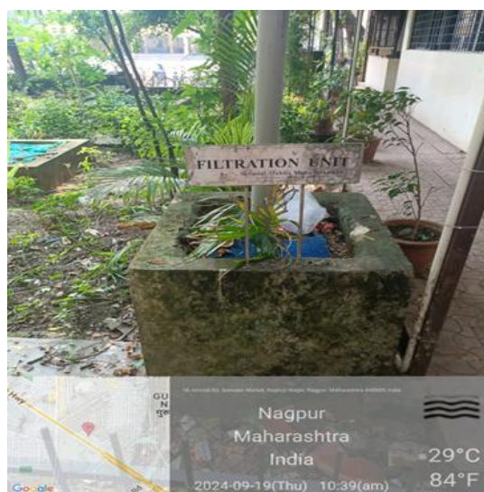
Rain water harvesting pipe
