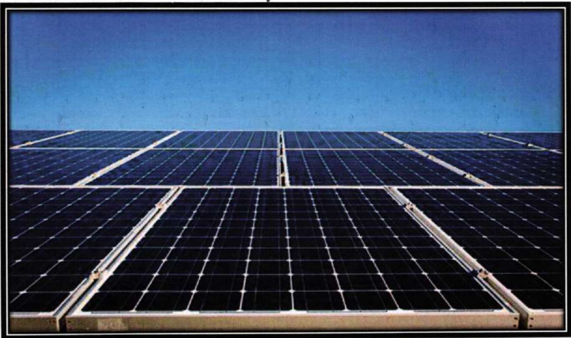
Solar PV system installed at college terrace
